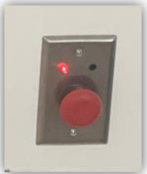
Keycard access labs Emergency door lock
